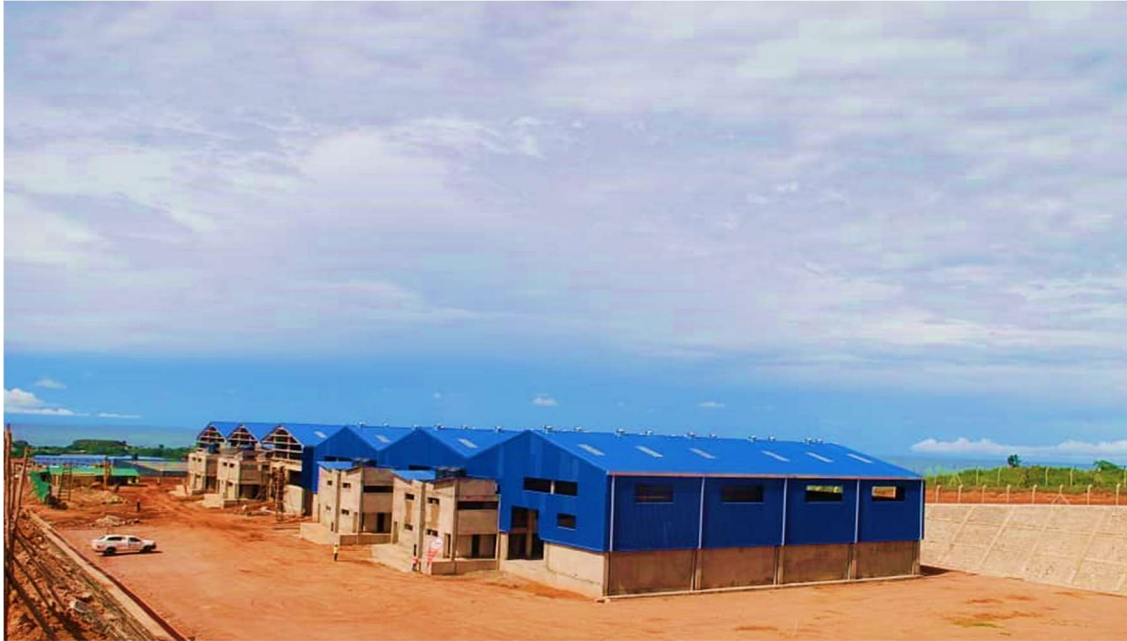
Progress of construction works at Entebbe International Airport Free Zone, within the precincts of Entebbe International Airport
